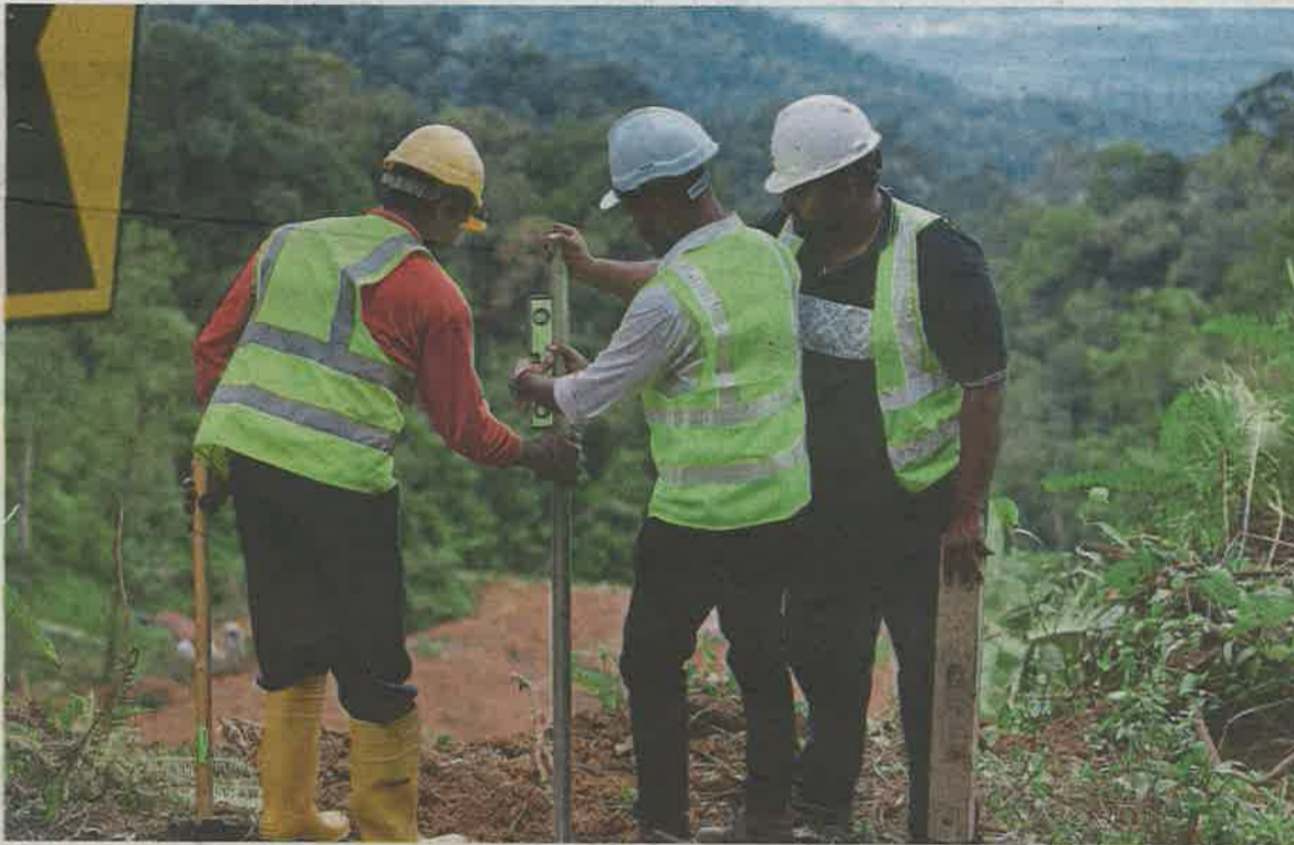
Early warning: Contractors installing a 'Real-Time Monitoring Device' at the Father's Organic Farm landslide site to detect soil movement in the area. — RAJA FAISAL HISHAN/The Star
